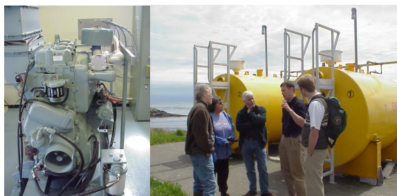
Figure 1: Race Rocks Diesel Generator and Tanks
